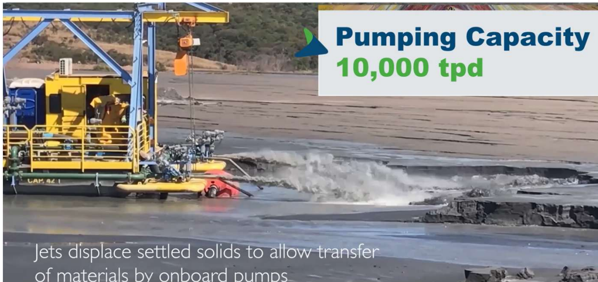
Onboard propulsion system using Goodwin Pumps and Intelligent Control System
